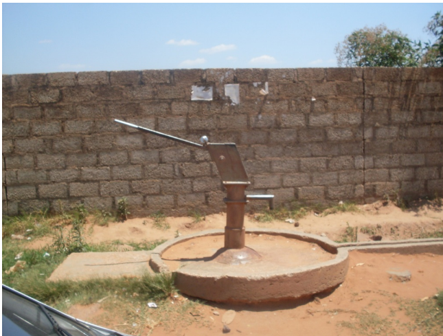
Broken down borehole as we entered the community which had been locked
